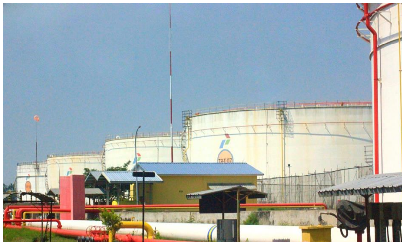
Gambar 1.2. Tangki BBM Fuel Terminal Tuban
